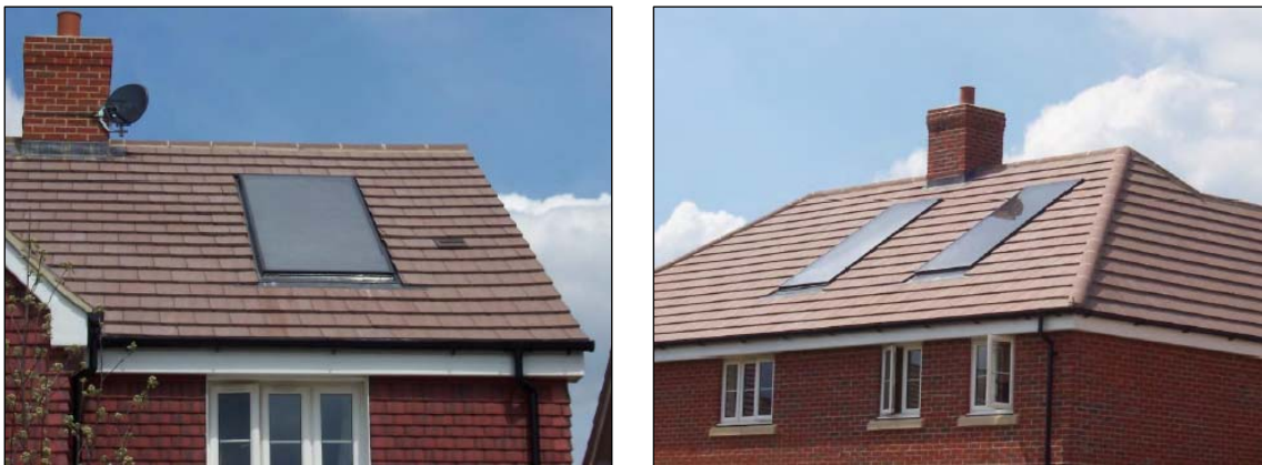
Flush mounted solar panels
