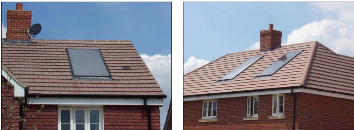
Flush mounted solar panels
