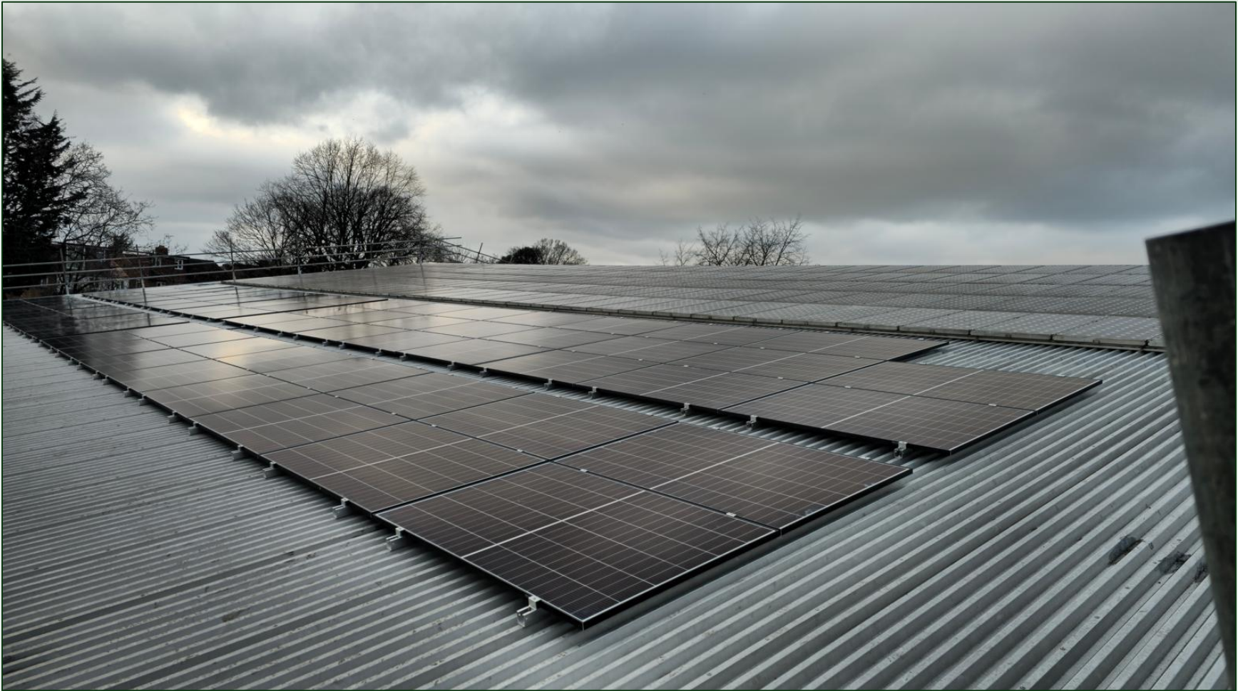
4.6. Figure 10: Solar Panels at Sunbury Leisure Centre installed March 2026
