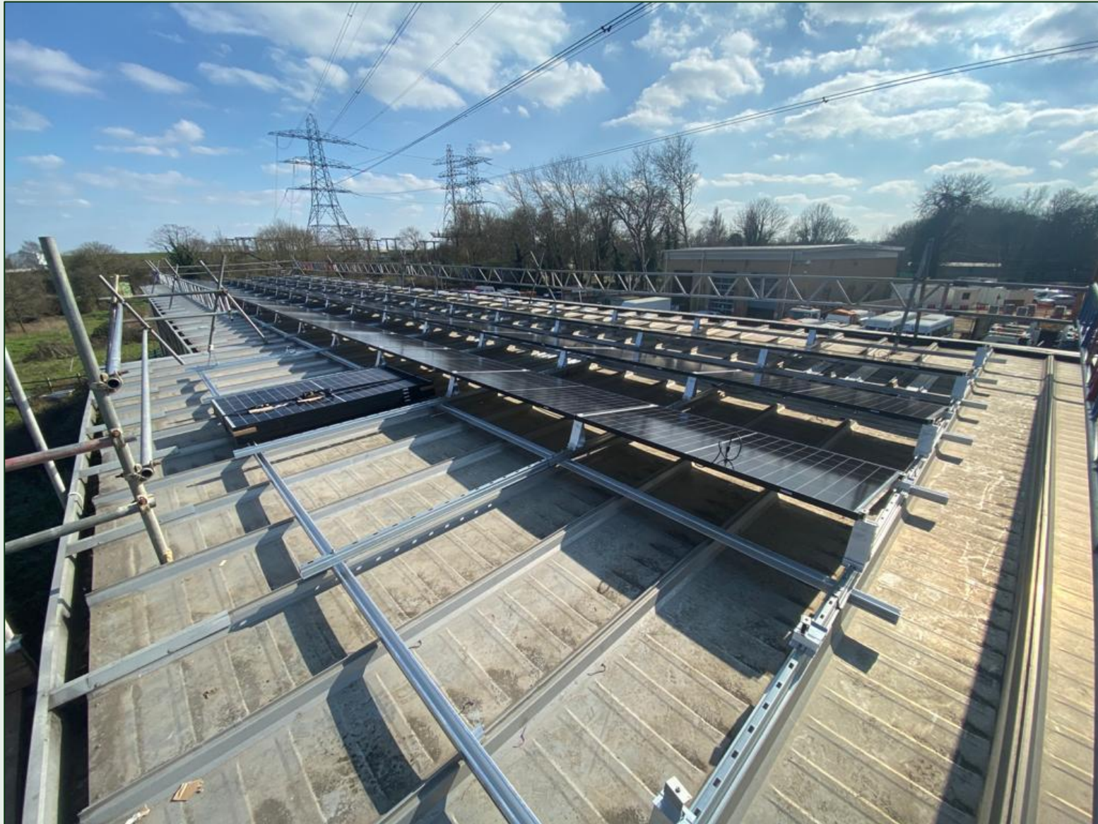
5.7. Figure 11: Solar Panels at White House Depot
